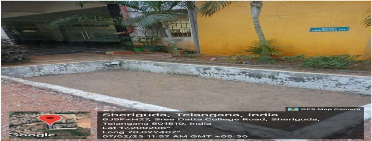
Rain water harvesting pit
