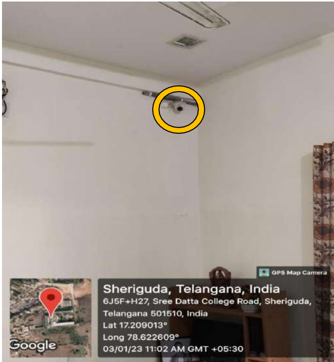
CCTV in the principal room
