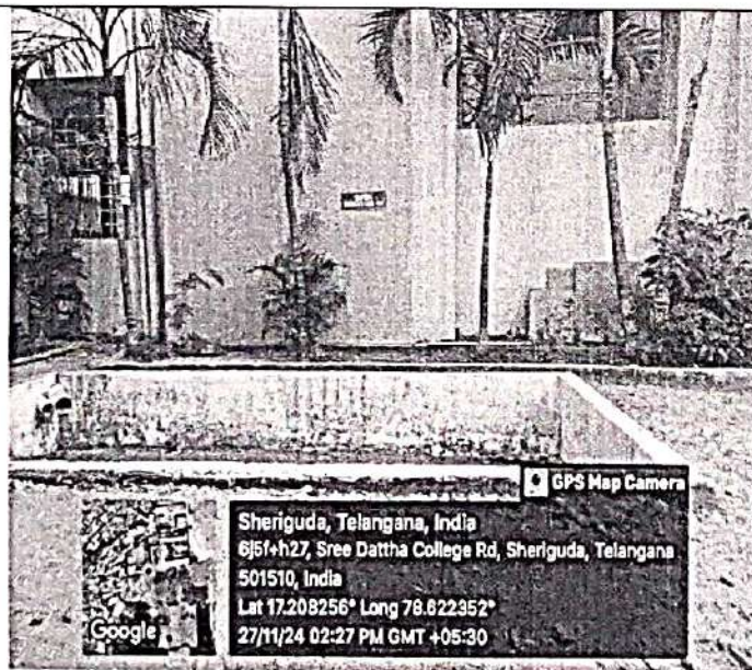
Rain Water Harvesting
