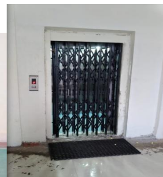
elevator for disable
